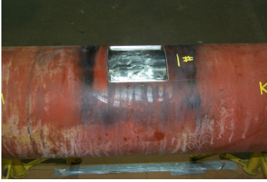
Defect - 6.5" x 6.5" x .300" Deep
