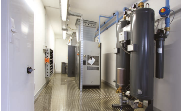
▲ Container with compressors, desiccant dryer, filter and oil-water separator Application: Brake tester for rail vehicles
